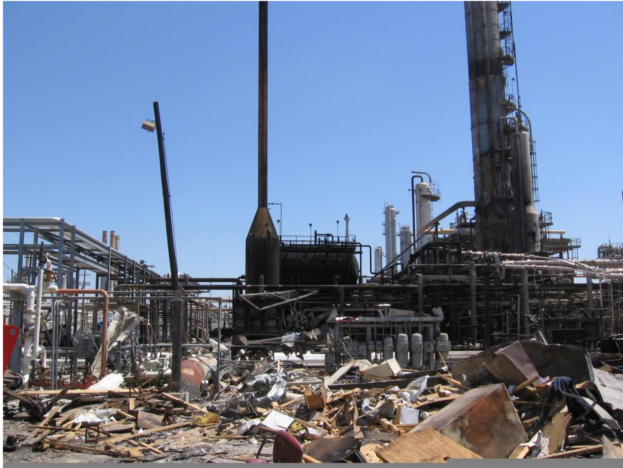
CSB (2007), "Investigation Report of Refinery Explosion and Fire, BP Texas City, Texas"
